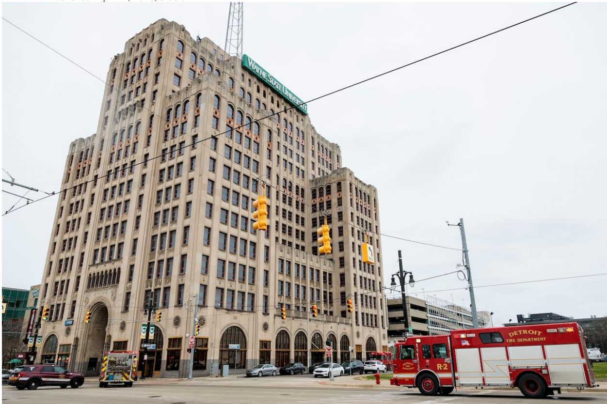
Damage from a rooftop HVAC fire can be seen to Wayne State University's Maccabees Building, 5057 Woodward Ave. in Detroit on Wednesday April 1 2026.MLive.com
